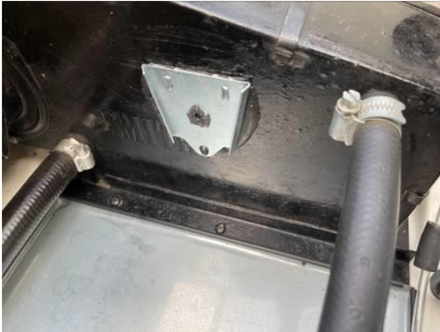
Not the smartest heater box in the world but it will get a refurbishment one day.
